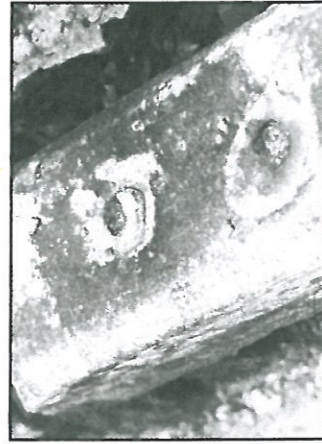
△ It is often possible to see where the railings once were. This picture shows the remains of some railings where they were cut level with the stone footings. You can also see the lead in which the railings were set.
